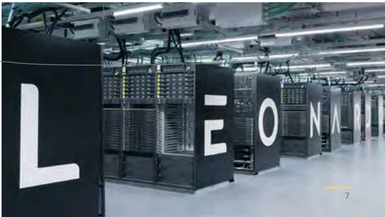
LEONARDO - BOLOGNA ITALY - 2022 Heating/cooling system
