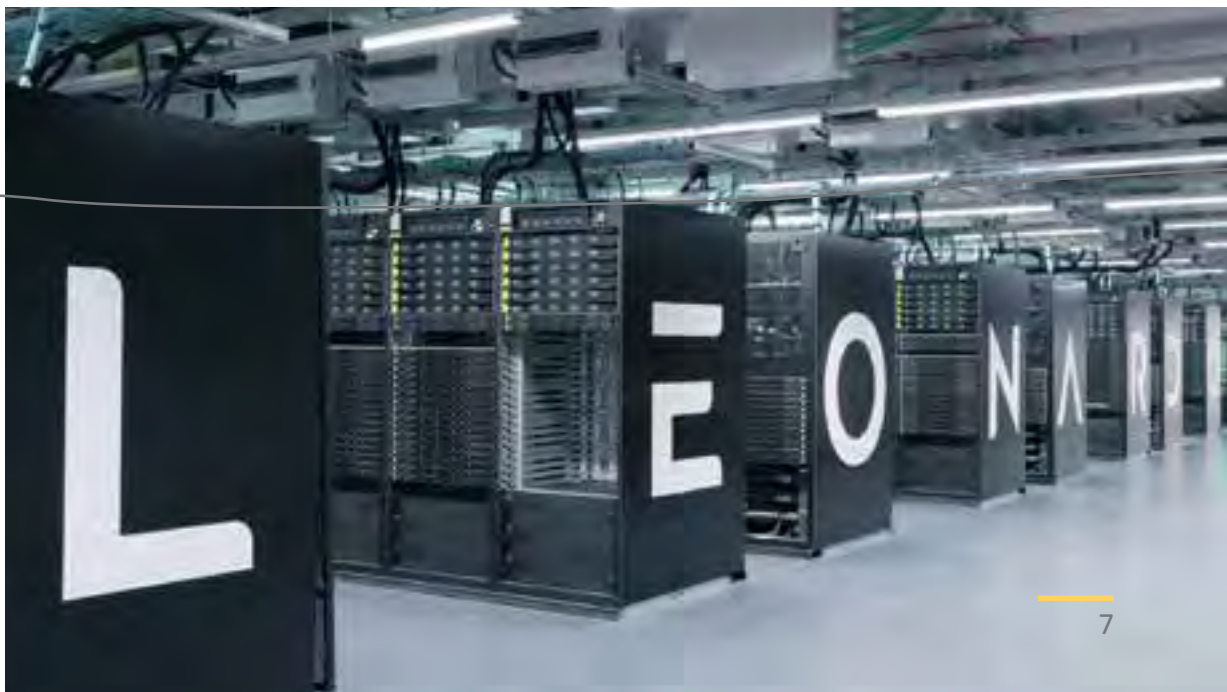
LEONARDO - BOLOGNA ITALY - 2022 Heating/cooling system
